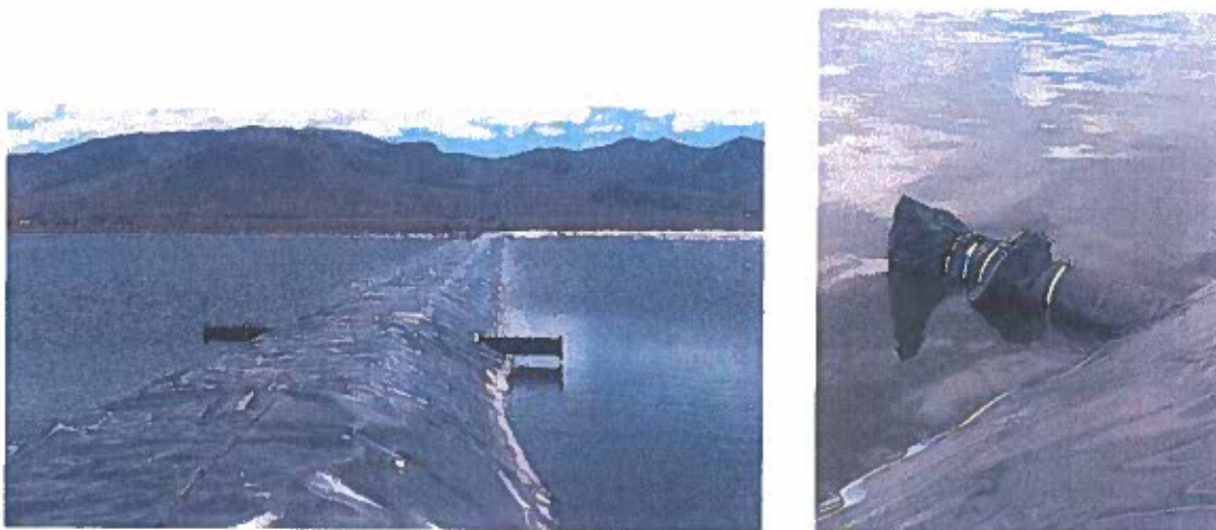
Figure 1: Pipe isolation of outlet pipes (left) and north pond inlet pipe (right)
