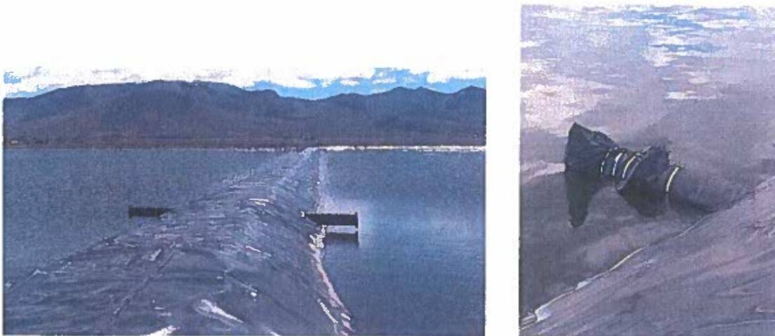
Figure 1: Pipe isolation of outlet pipes (left) and north pond inlet pipe (right)
