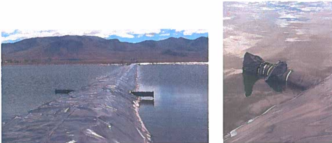
Figure 1: Pipe isolation of outlet pipes (left) and north pond inlet pipe (right)
