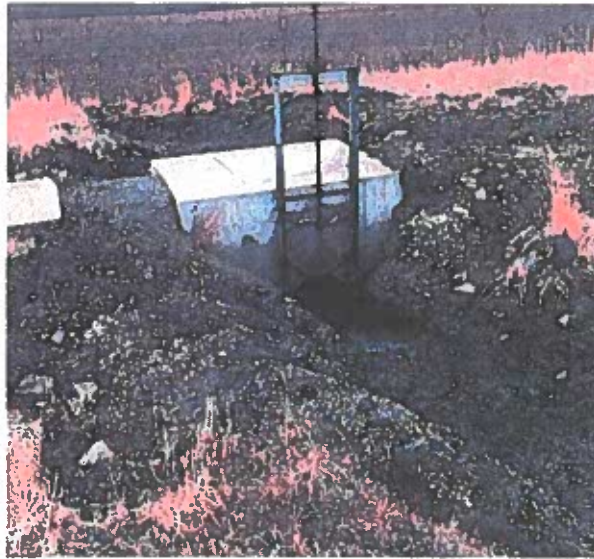
Figure 1: Photo of the tailwater diversion box shows maintenance performed to ensure that runoff from the land application area is returned to the WWTF.
